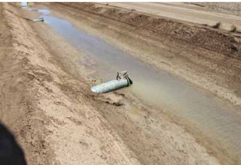
Pipe through the bank with valve mechanism.
